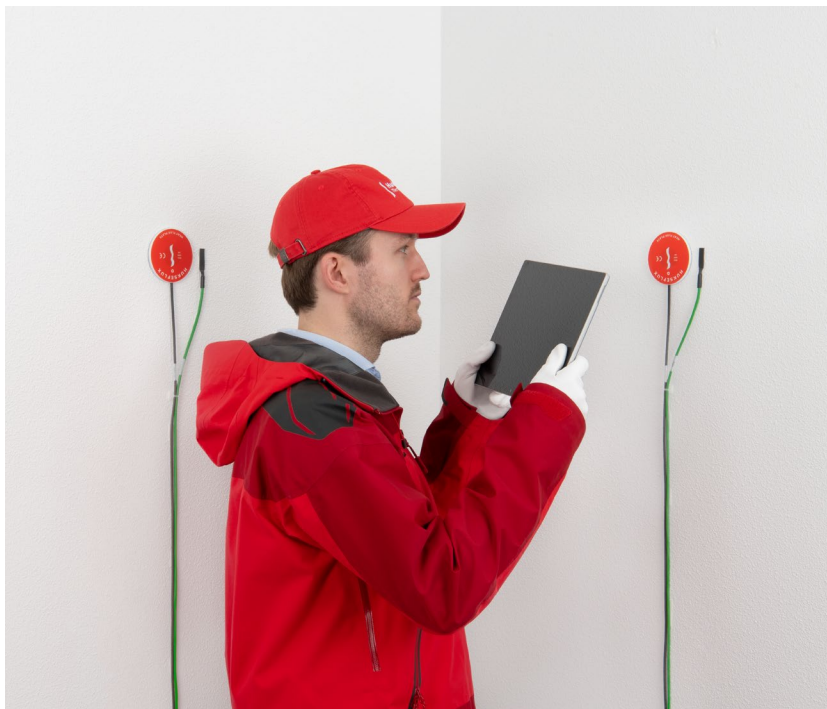
Figure 2.1 HFP01 heat flux sensor and TC mounted on a wall.
