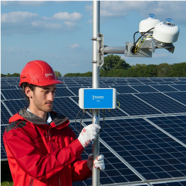
Figure 7 Two SR300-D1 pyranometers that are connected to the SPD01 Surge Protection Device. With the optional SPD01, you can upgrade surge immunity to Level 4.
